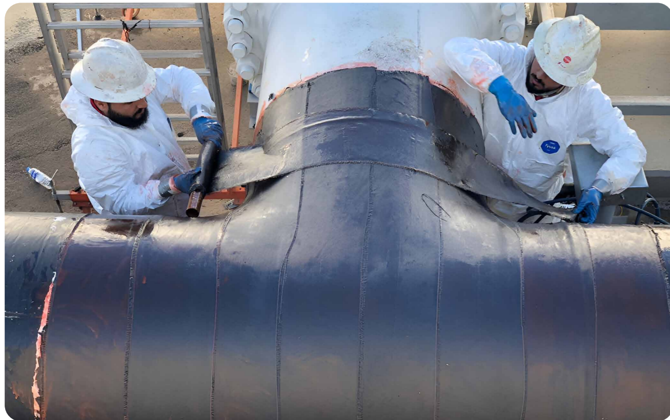
A large pipeline in Iraq with multiple areas of external corrosion at the intersections of a T component was rehabilitated using Revowrap, eliminating the need to replace the piping system.
