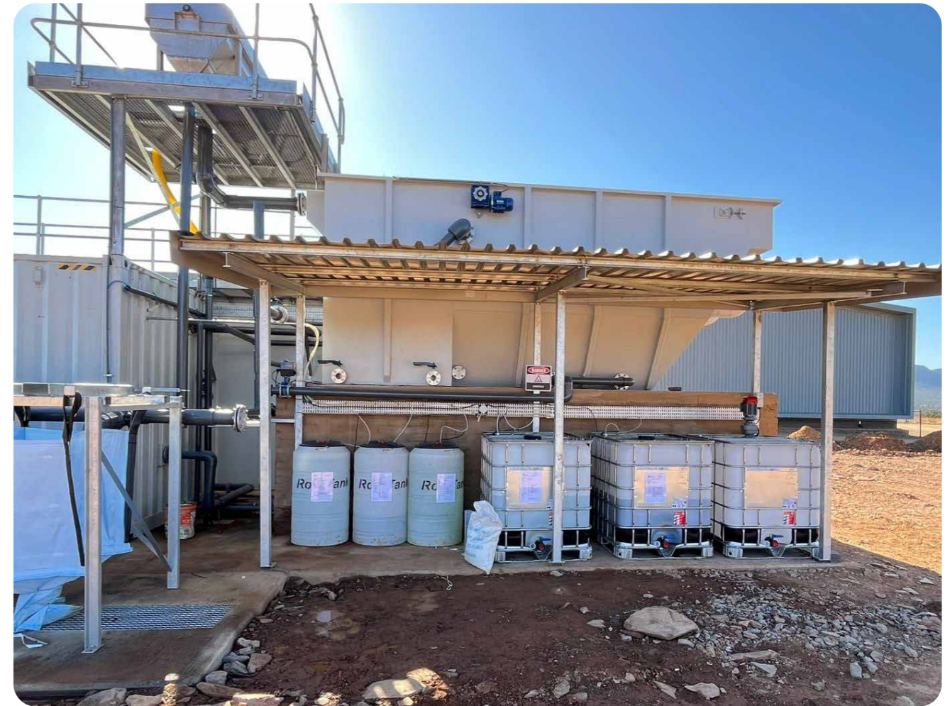
The completed DAF, featuring a flotation tank, chemical dosing tanks and MBBR bioreactor
