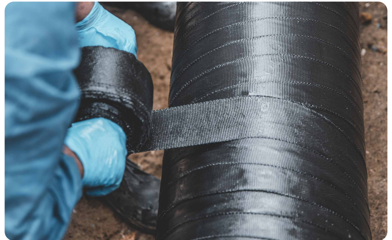
A 12" white oil pipeline with internal corrosion was safely excavated, repaired using Revowrap, and restored to service with reinforced structural integrity and corrosion protection.
