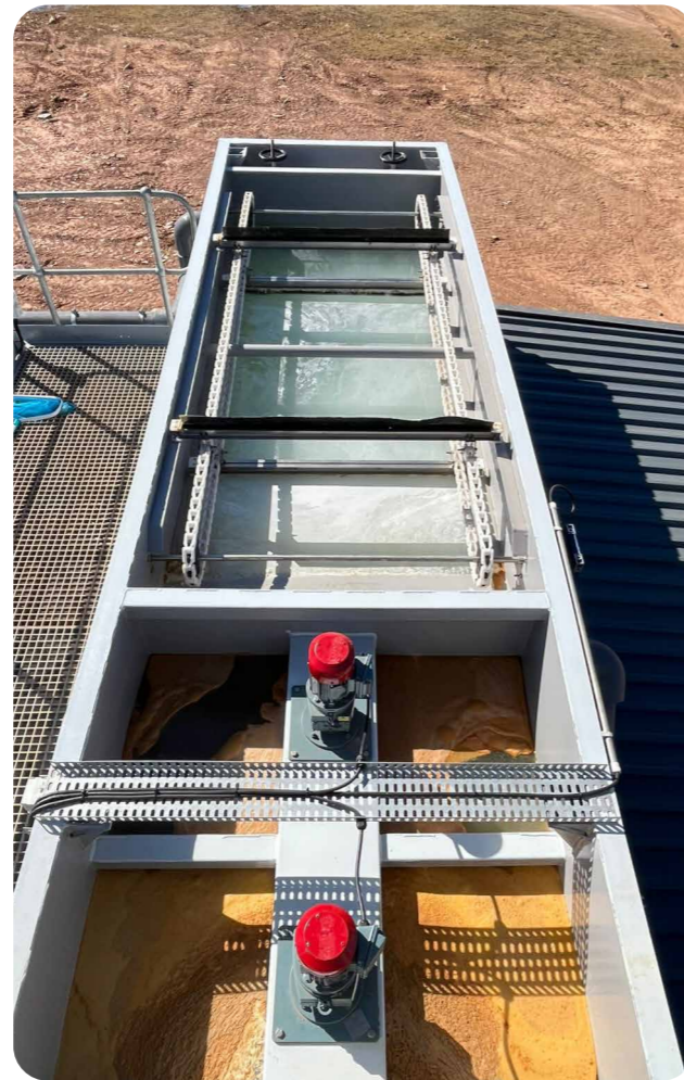
Top view of the DAF in operation, showing the flocculation tanks with mixers and the flotation chamber with scraper flight
