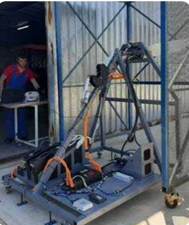
JS2 RES System Ground test bench
