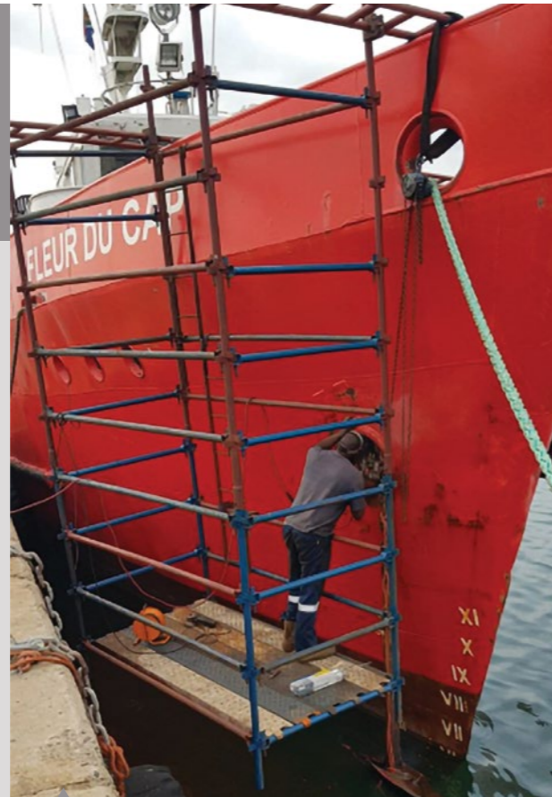
A Macc Marine employee working on a docked utility vessel. The company is now in a formidable position to secure future steelwork contracts and projects having secured IACS certification.
